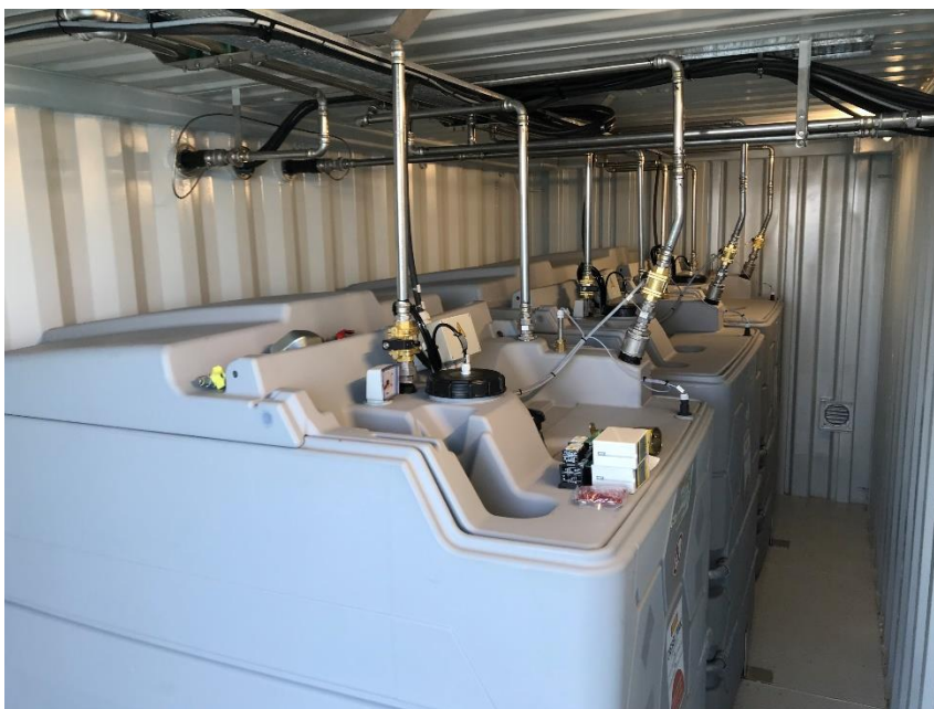
Caption: The system has an overall capacity of 15,000 litres.
