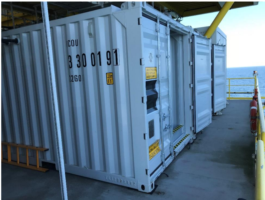
Caption: The newly installed tank facility consists of two offshore containers (20 ft) fitted with 3 CUBE tanks each.
